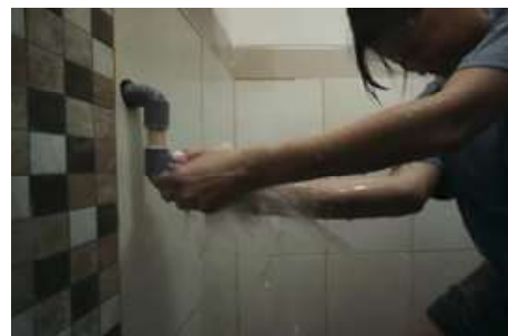
Figure 4 The back bathroom faucet has come loose.
